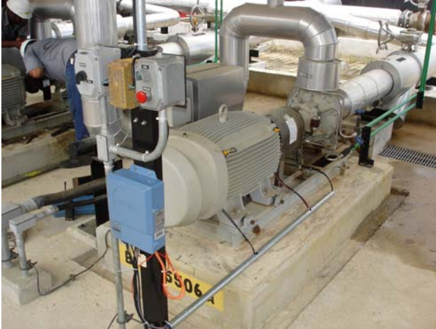
A typical large commercial pump motor unit.
