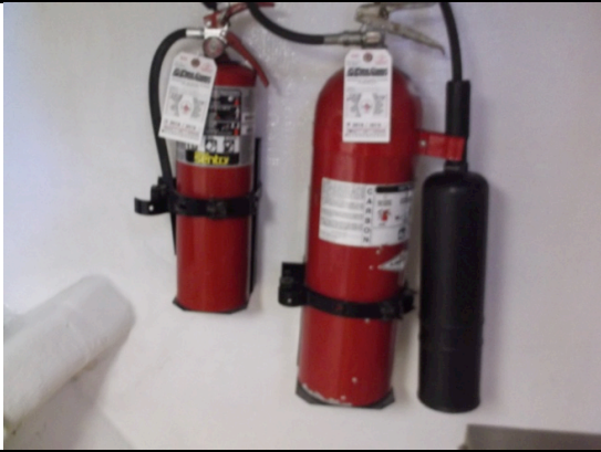
17 Typical Portable Fire Extinguishers
