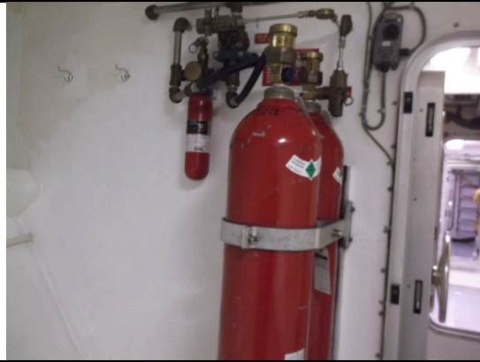
18 Fixed Firefighting System
