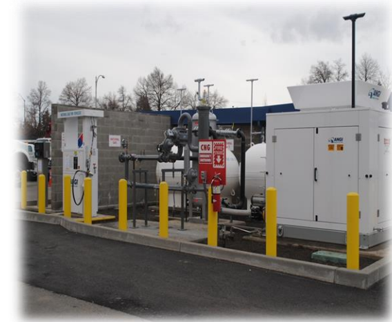
Mission Avenue Refueling Station - Spokane
