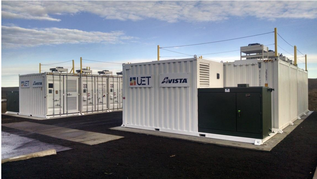
Turner Energy Storage Project, Pullman, WA
