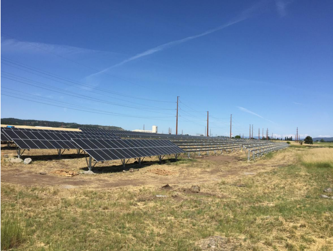
Boulder Park Community Solar Project
