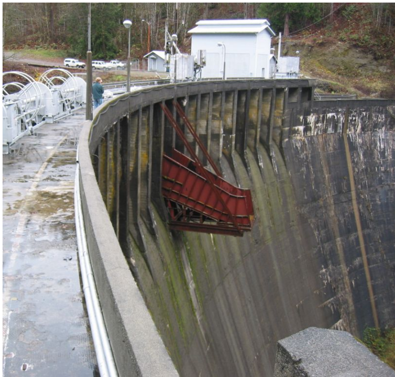
Photo 4 – AC hoist cart near center of photo, DC hoist cart at right edge of photo. Steel chute directs debris away from face of dam. Lower Baker Dam
