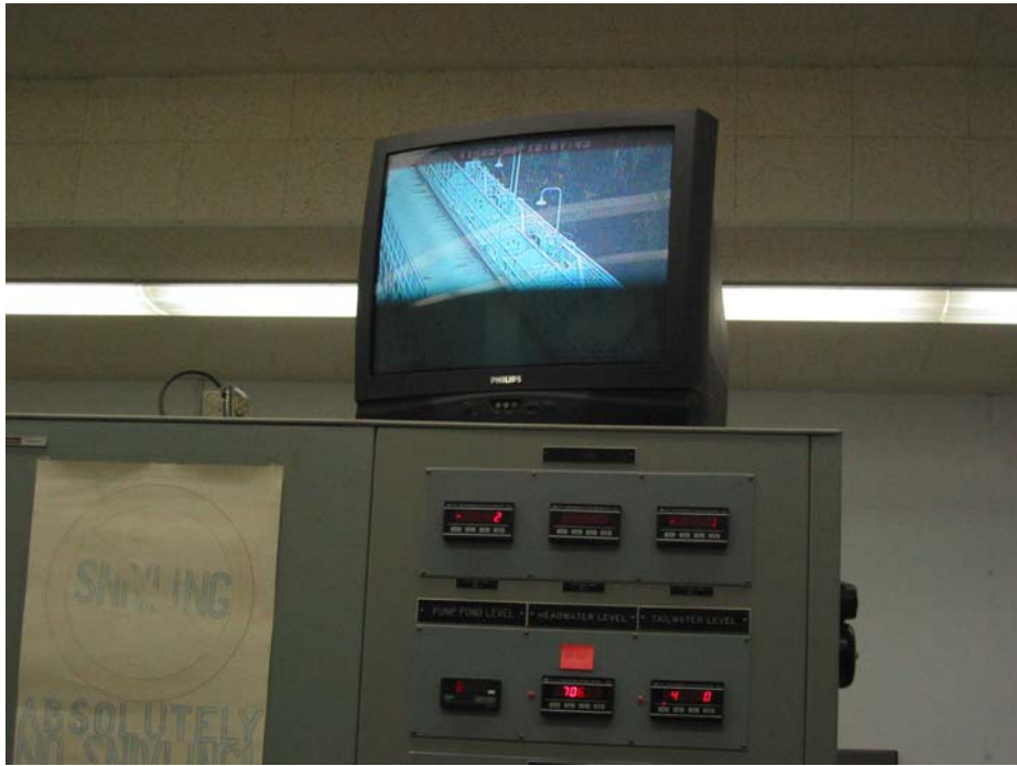
Photo 7 – Video monitoring of spillway gates from Upper Baker Powerhouse to assist in remote gate operations.
