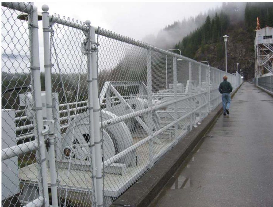
Photo 6 – Thirty ton capacity, bridge-mounted, electrical drum hoists are used to lift the three radial gates at Upper Baker Dam
