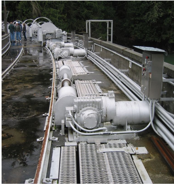
Photo 5 – Fixed electrical driven hoist equipment used to lift 13 of the 23 Lower Baker spillway gates. Manual switchbox appears at right edge of photo.
