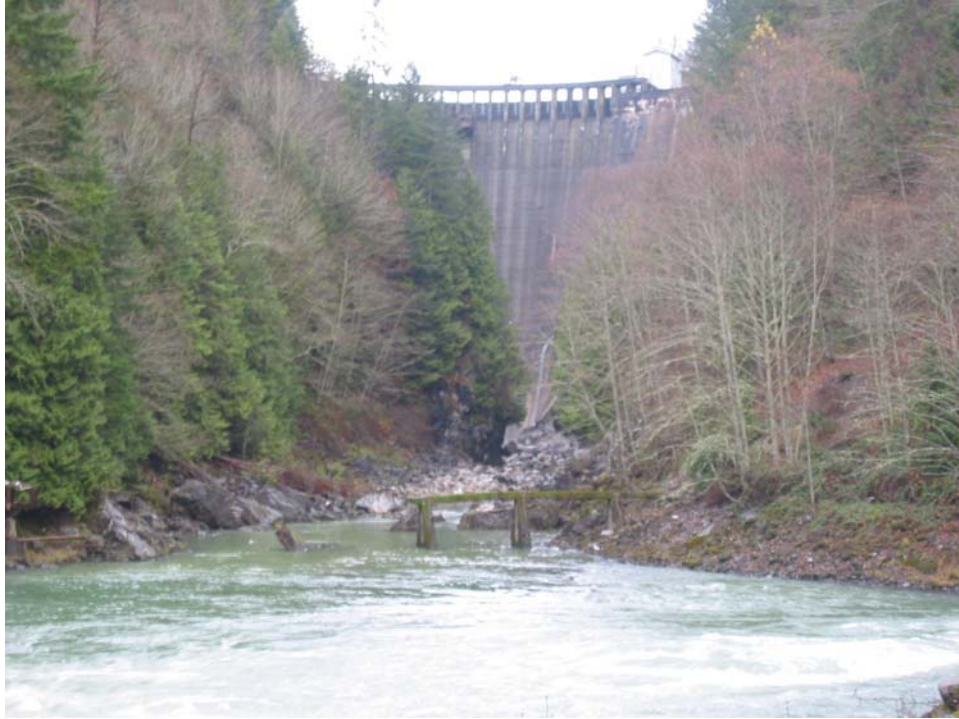
Photo 1 – Looking upstream towards the downstream face of Lower Baker Dam (photo taken from vicinity of the powerhouse)
