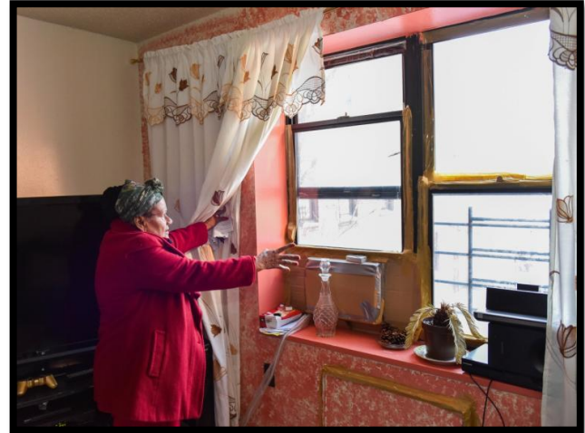
Resident reveals the duct taped windows in her Claremont Houses apartment in the Bronx, NY.
