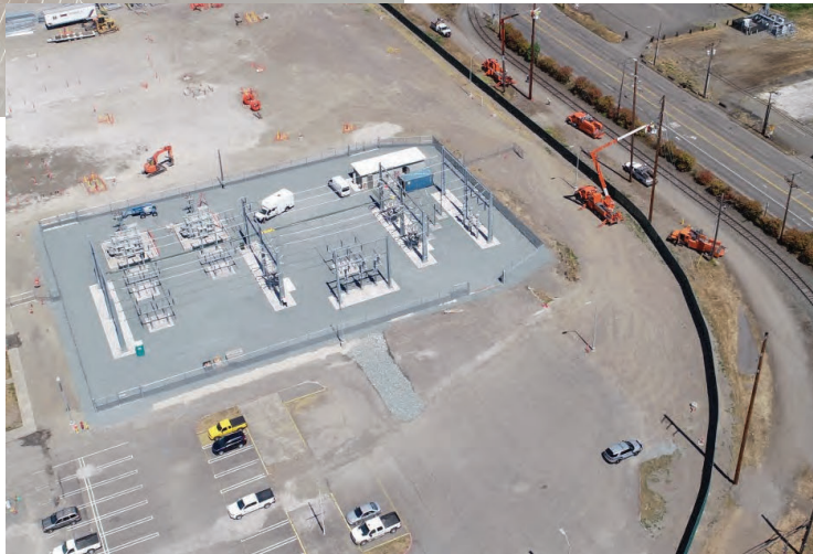
Completed Tacoma Power substation
