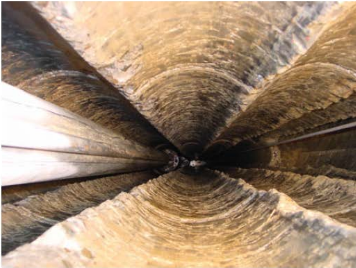
Exhibit Alt 2D-4: Downhole photograph of overlapping secant pile drill holes, Arapuni Dam (Amos and others, 2008)
