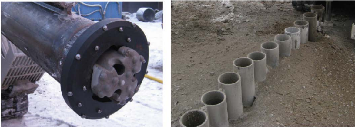
Exhibit Alt 2D-6: RD pile bit and downhole hammer (left) and view of top of piles after installation (right) (Uotinen and Jokiniemi, 2012)
