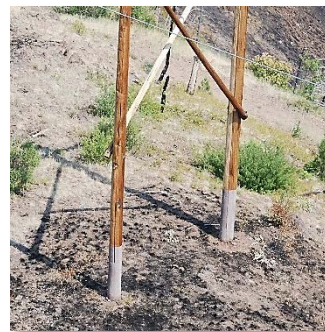
Fire resistant paint protected a structure from a recent fire
