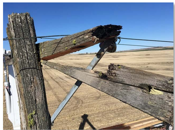
Crossarm tracking fire damage
