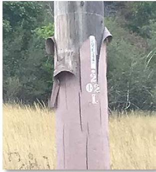
Fire resistant paint tends to crack or peel after about 5 years, so the Company is moving to wire mesh wrap.
