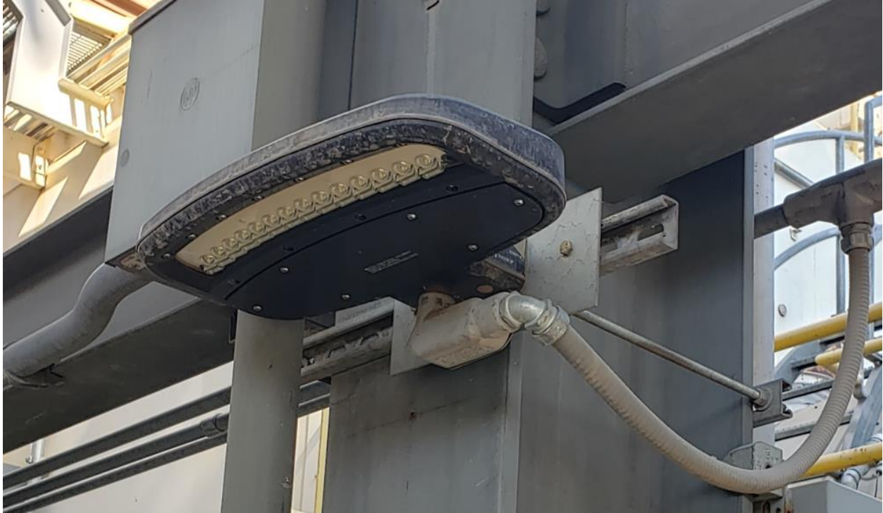
Figure 3: Outdoor LED Lighting on Unit 2 with Light Sensor
