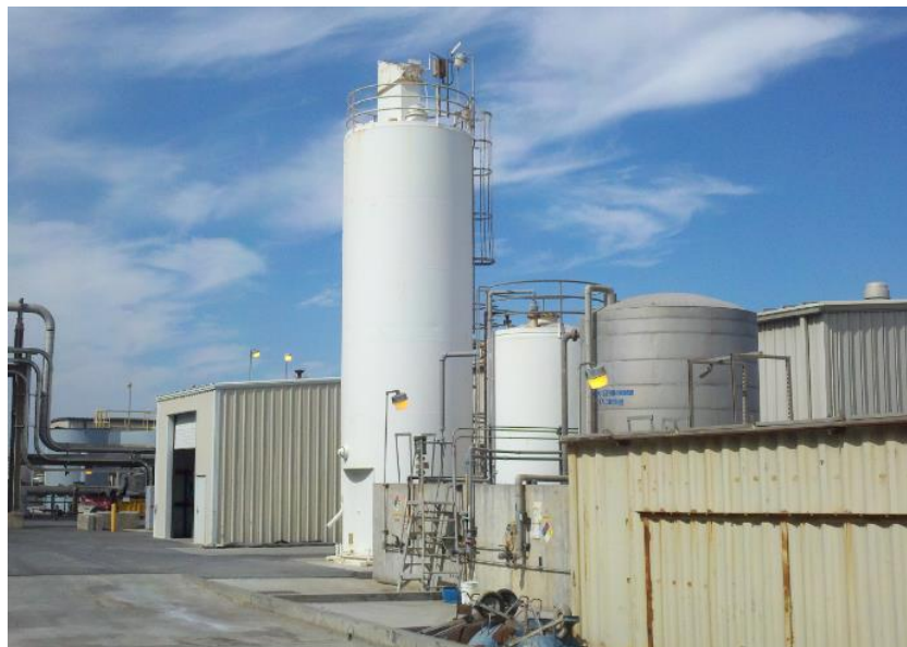
Figure 3: High Pressure Sodium Lighting Outside Demin Building
