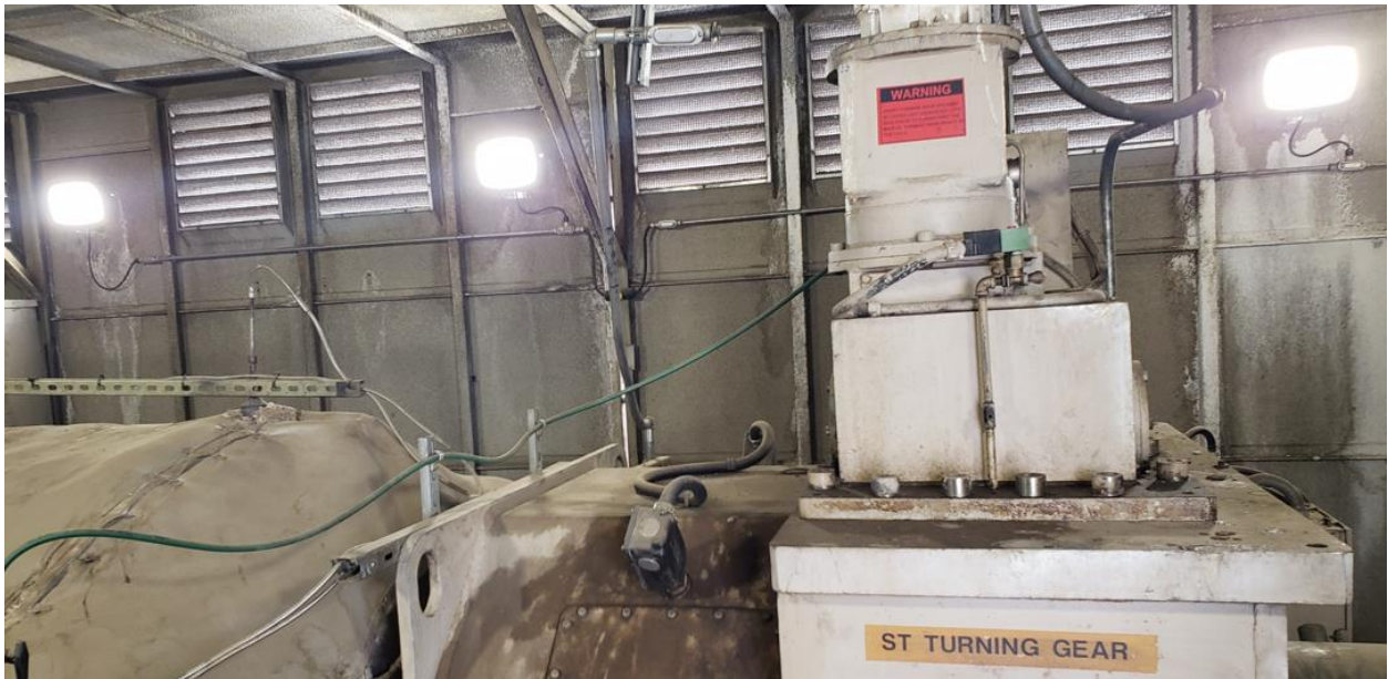
Figure 5: Unit 1 Steam Turbine Building LED Lighting
