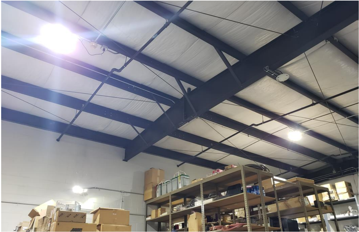
Figure 4: Maintenance Building LED Lighting with Occupancy Sensors
