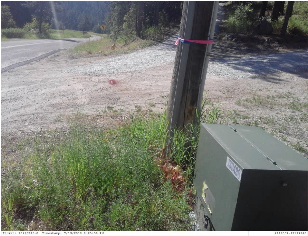
Attachment C: Picture of electric locate marks at pole located at 42994 S Loon Lake Road and marks going east.
