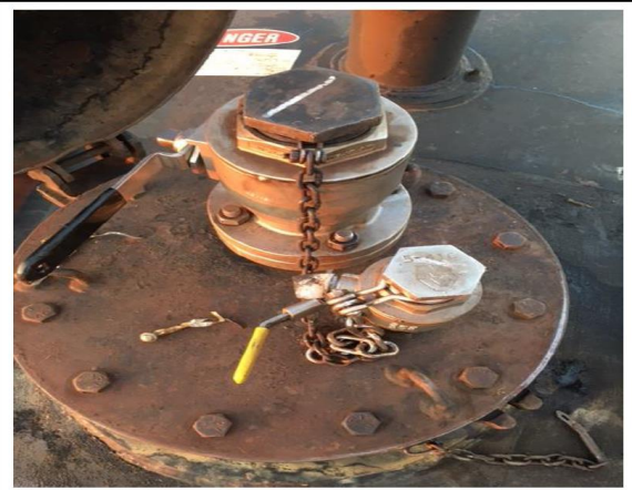
Photo 6: Flange bolts found less than finger tight.
