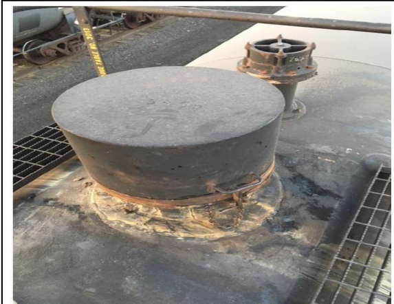
Photo 5: Product visible around manway.
