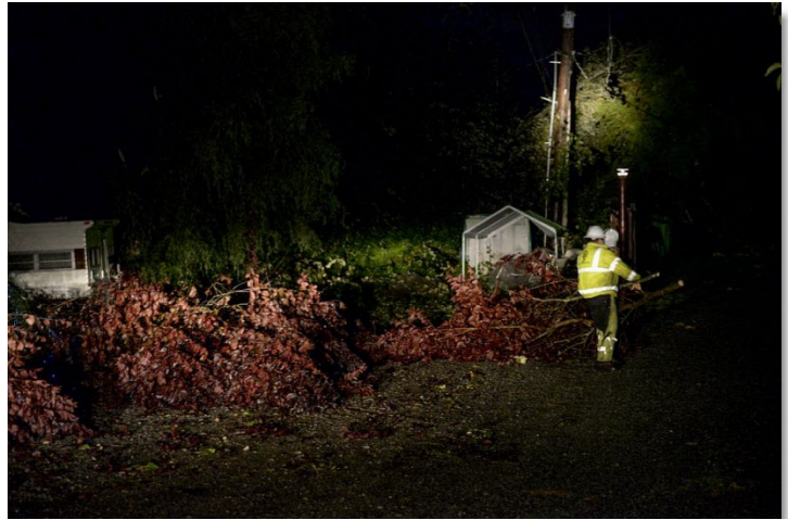
Puget Sound Energy crews worked through the night to restore power to thousands of customers.
