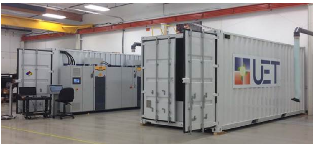
Uni.System grid-scale batteries from UniEnergy Technologies
