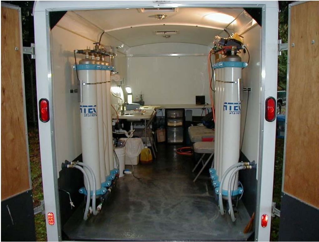
Picture above shows the interior of the pilot plant trailer from the rear. The sample outlets and the analytical equipment are on the desk in the front of the trailer.
