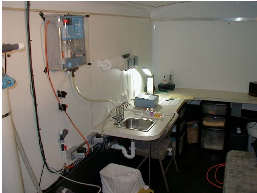
The front one-half of the trailer is shown above. The instrument foreground on the wall is an in-line chlorine analyzer. The smaller boxes on the wall above the light are electronic flow meters used to monitor cumulative as well as instantaneous flow for each treatment train in the pilot plant.
