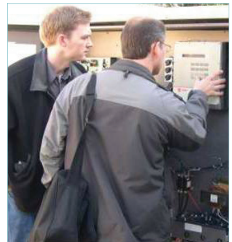
Data in a digital format enables the analysis of energy use which in turn identifies opportunities to adjust building system performance for optimization
