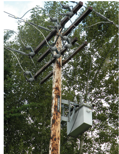
Recloser on PSE power pole
