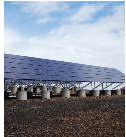
Demonstration solar array at PSE's Wild Horse Wind and Solar Facility
