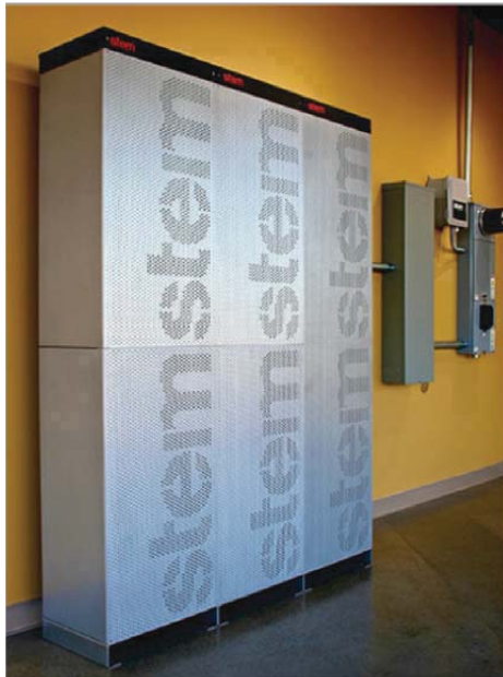
54 kW/54 kWh commercial customer-sited lithium-ion battery.
