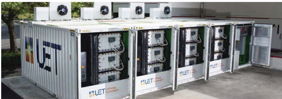
1 MW/3.2 MWh distribution-connected vanadium redox flow battery.
