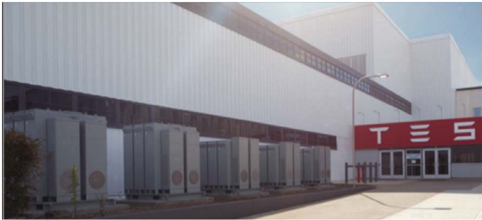
1 MW/2 MWh customer-sited lithium-ion battery.
