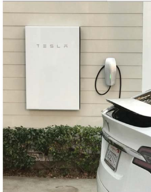
7 kW/14 kWh residential customer-sited lithium-ion battery.
