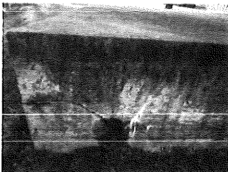
North Side Large Storage Tank
