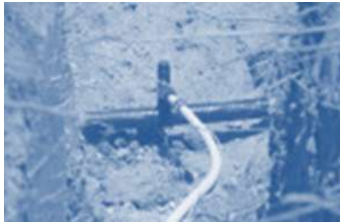
Figure 4. Typical polyethylene service tapped from a steel main.
