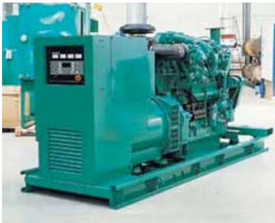
Figure 2-19. Reciprocating Engine (Madison Gas and Electric, 2015)
