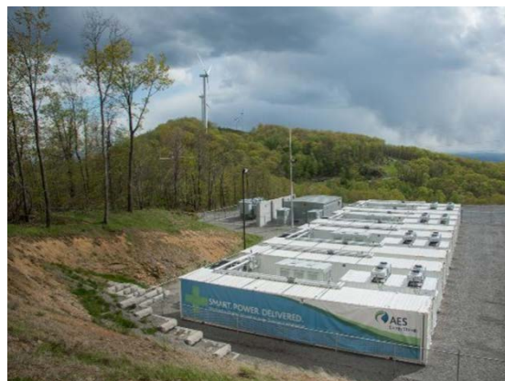
Figure 2-22. Battery Storage (Wood, 2014)
