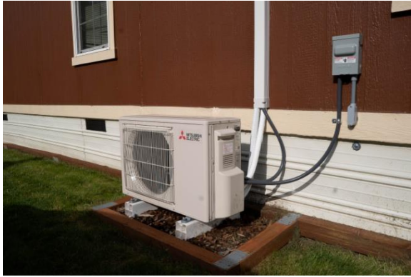
Figure 1. Demonstration DHP Outdoor Unit
