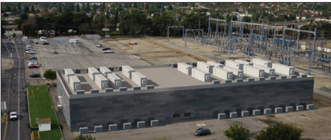
Proposed 100 MW/400 MWh transmission-connected battery.
