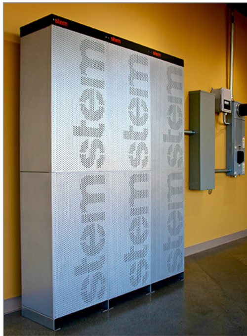
54 kW/54 kWh customer-sited lithium-ion battery.
