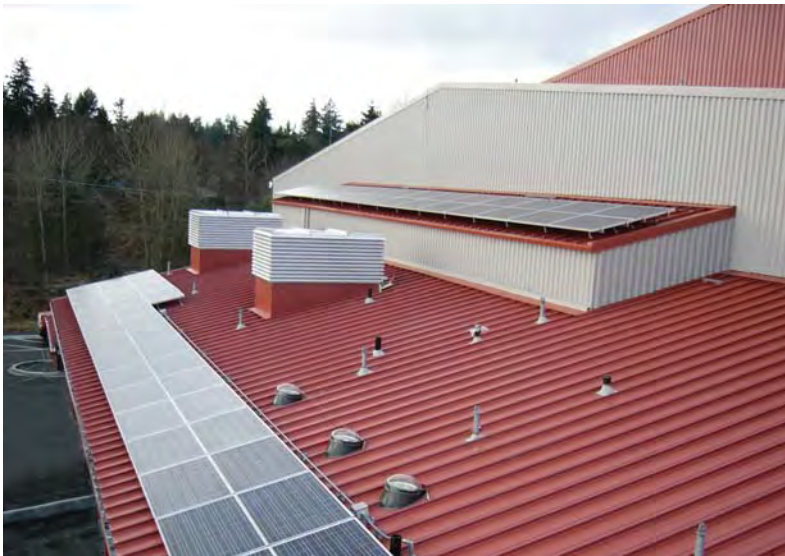
Solar panels on the south roof of the Shoreline Recycling and Transfer Station, one of the many green features of the building.
