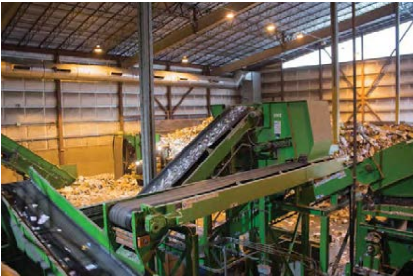
Recology CleanScapes materials recovery facility
