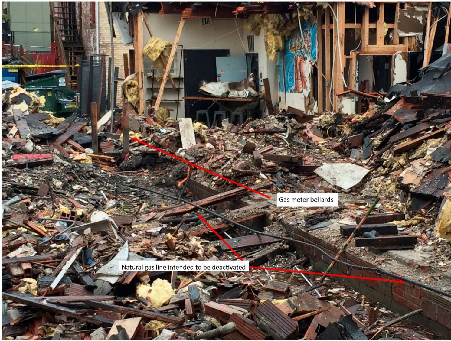
Image 23. Photo depicting location of service line involved in explosion.
