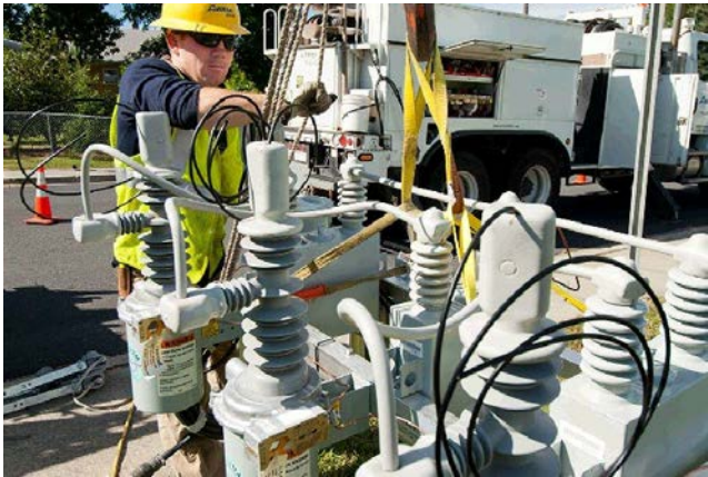
Capacitor – Line Device
