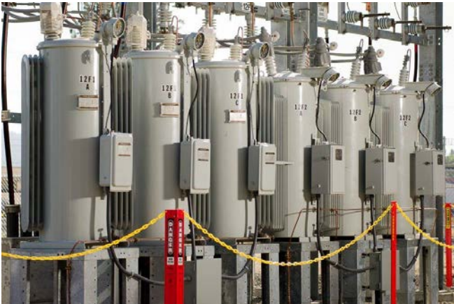
Substation Voltage Regulators
