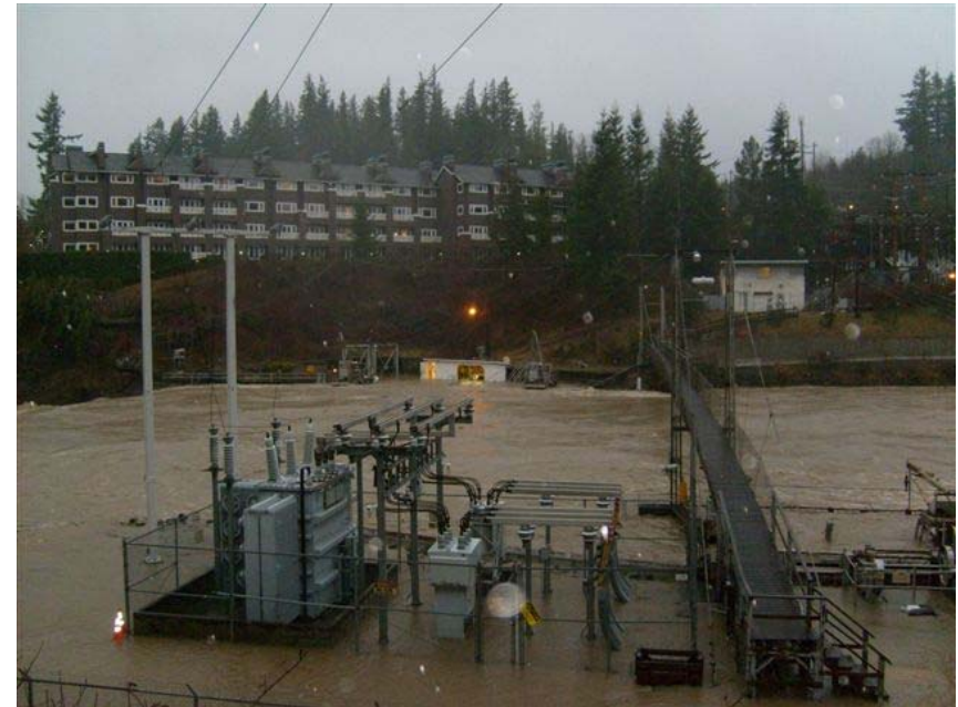
PSE's Snoqualmie Falls generation substation is submerged in water during the January 7, 2009 flood. While a designed barrier protects the transformer, the substation damage included wet equipment, silt and erosion that undermined the site. ©PSE
