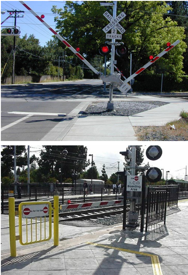
Figure 76. Pedestrian Automatic Gate Examples
