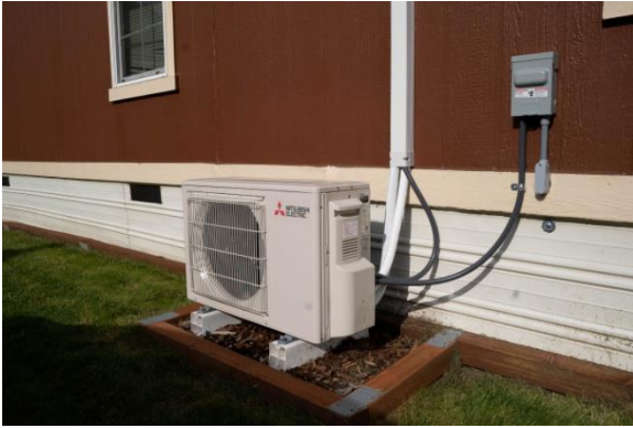
Figure 1. Demonstration DHP Outdoor Unit
