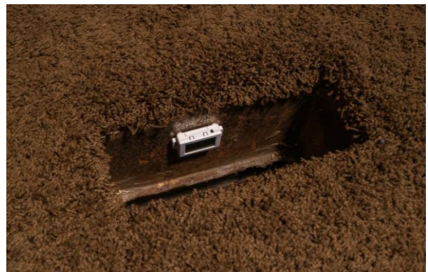
Figure 6. Temperature Logger as Installed in eFAF Duct-Register Removed
