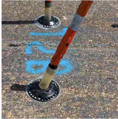
Figure A-4. Sample 2B Failure at 44 Impacts.
