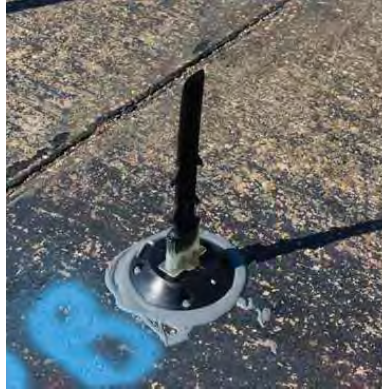
Figure A-14. Sample 7B Failure at 18 Impacts.
