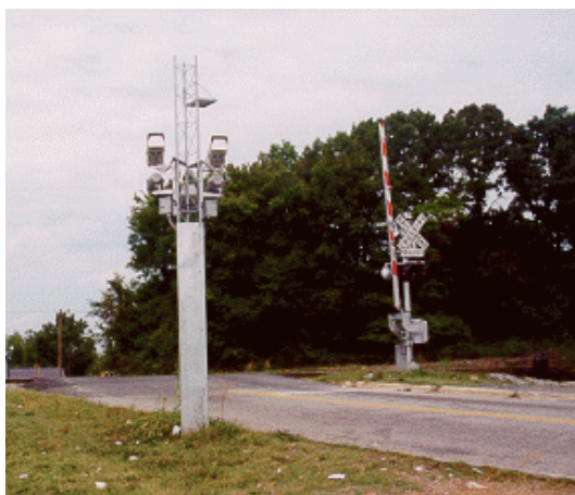
Figure 5. Photo Surveillance Hardware
