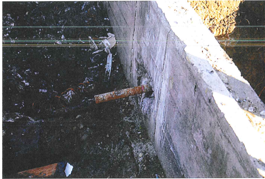
Photo 9: View of the gas fuel pipe entry into crawl space through east foundation wall. The vertical saw cuts in the concrete wall were made after the incident. Photo taken October 18, 2011, by Dennis Ritter, UTC engineer
