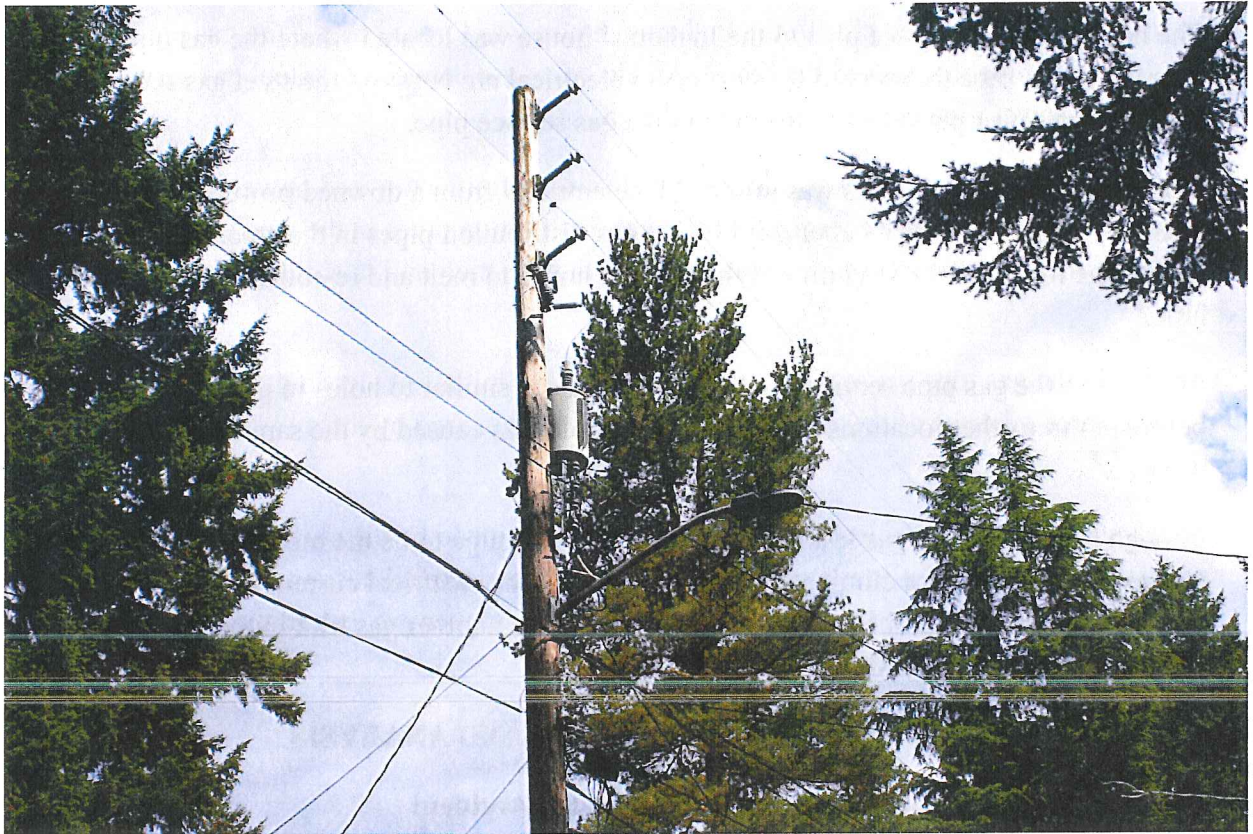
Photo 1: View of high voltage line (top of pole) near the intersection of N.E. 127 th Street and 10 th Avenue N.E. Photo taken September 30, 2011, by Kuang Chu, UTC engineer.
