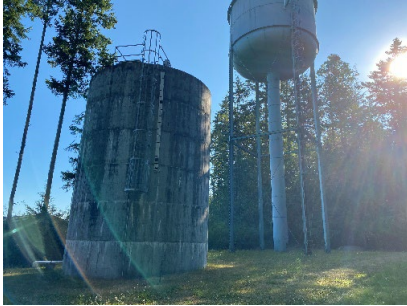
Tank 2 & 3 at Transfer Station
