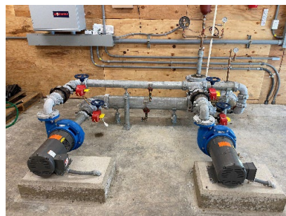
Booster Pumps in Transfer Station
