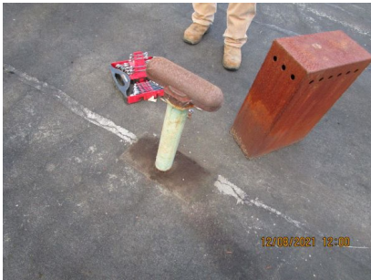
Large Storage Tank Vent
