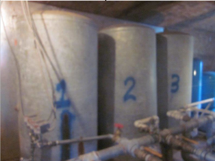
Lower zone pressure tanks
