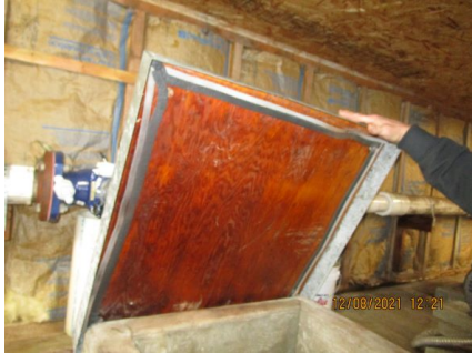
Large Storage Tank Hatch Gasket
