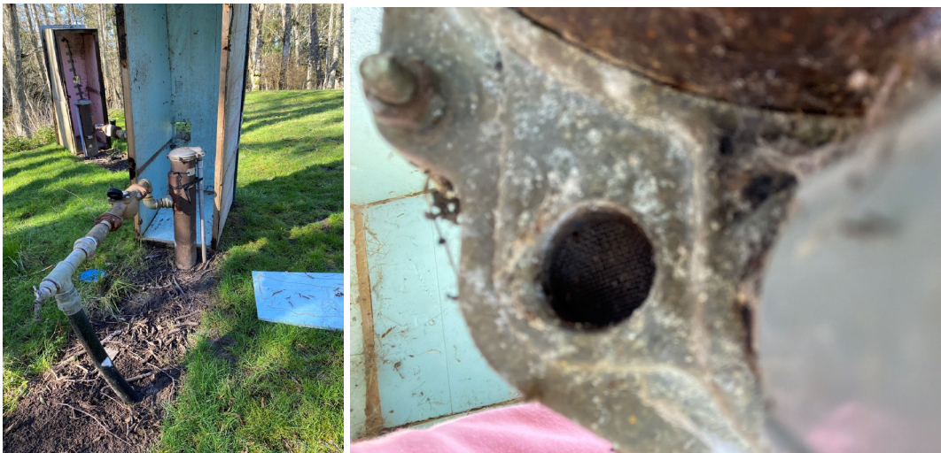
(L) Well #1 with sample tap and source meter (R) Screened vent on Well #1
