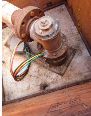
Well 1 With Sealed Wires
