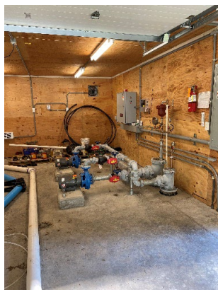
Booster Pump Transfer Station
