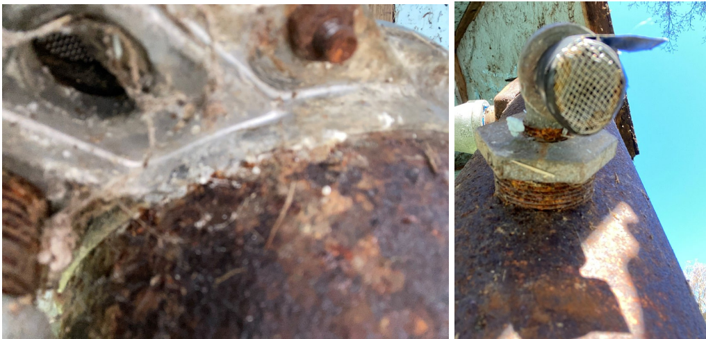
(L) & (R) Screened vents on Well #3
