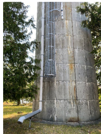
West St Storage (Tank 1)
