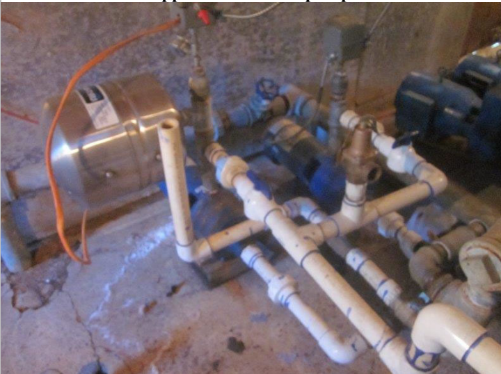
Upper zone booster pumps
