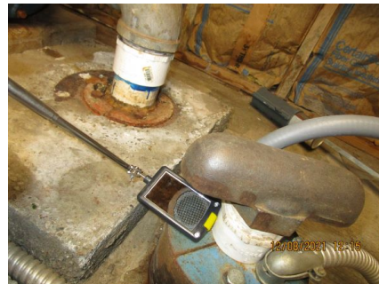
Small Storage Tank Vent
