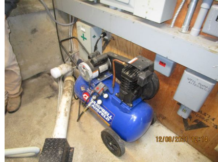
Oilless Air Compressor for Pressure Tanks
