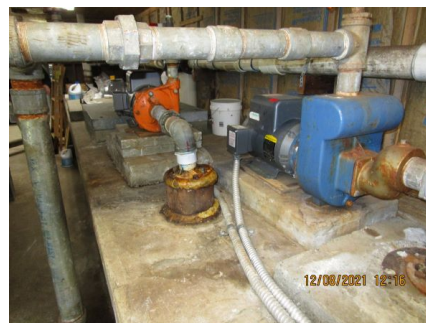
Booster Pumps for Small Storage Tank
