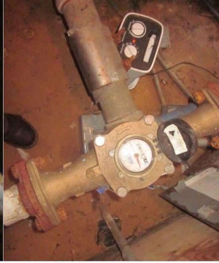
SO1 water meter
