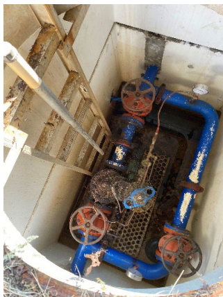
Altitude Valve controlling West St Tank water level
