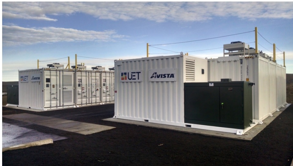
Turner Energy Storage Project, Pullman, WA
