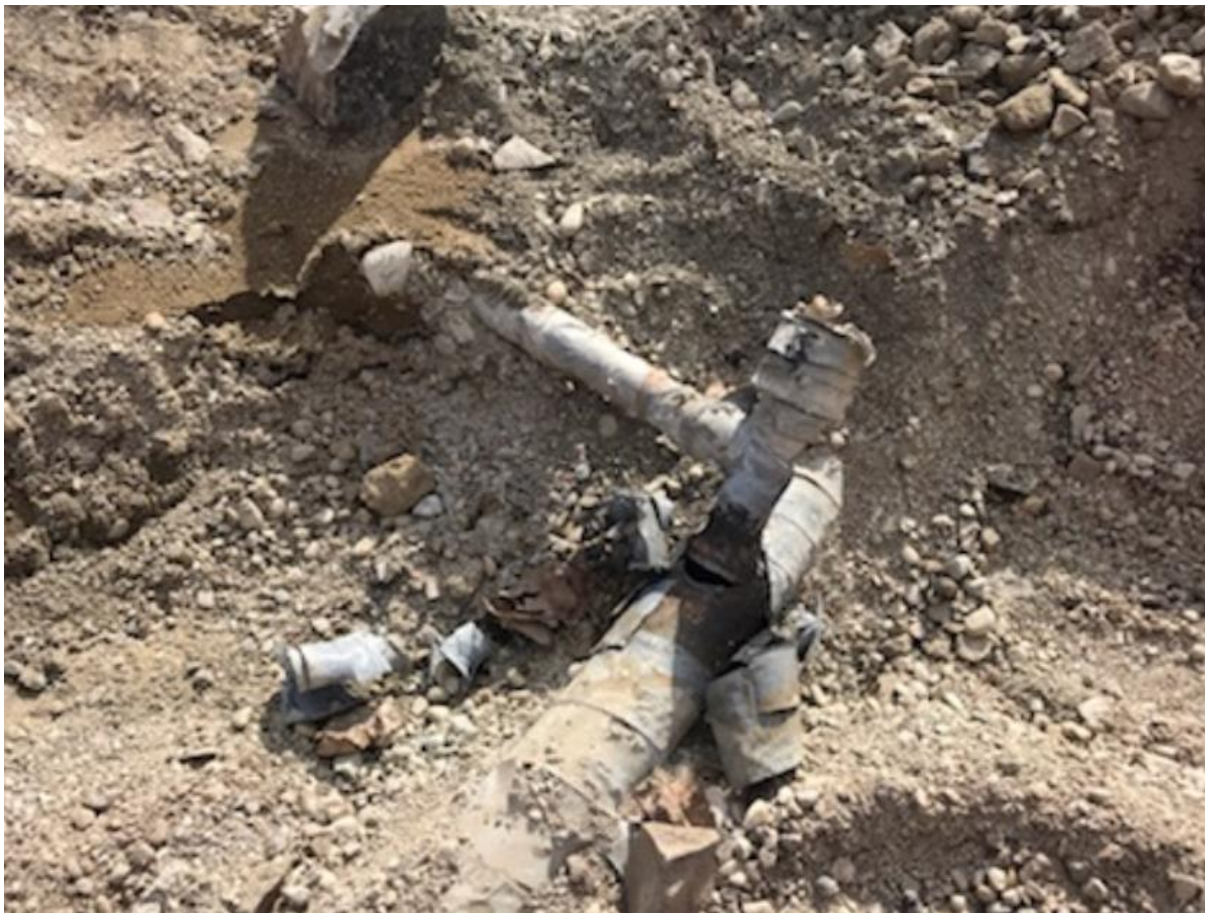
Attachment #4 – Close up picture of damage. Steel service tee broke off 2" steel main
