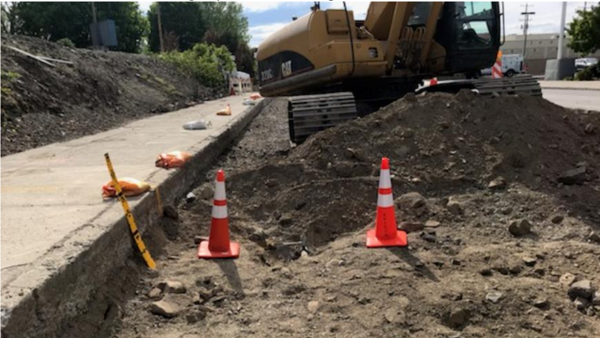
Attachment #3 – View of damage by trackhoe looking west on 3 rd Ave
