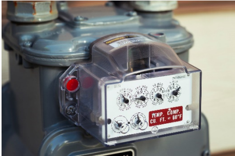
Residential natural gas meter
