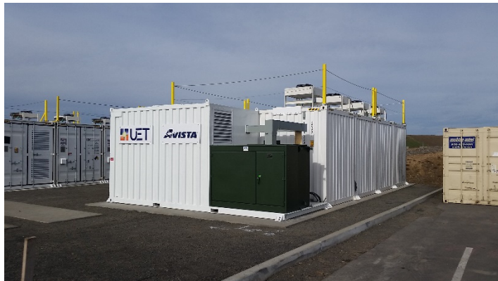
Vanadium Flow Battery as installed at the Turner facility
