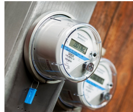
Electric smart meters
