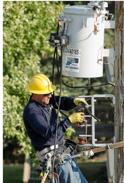
Installation of smart transformer
