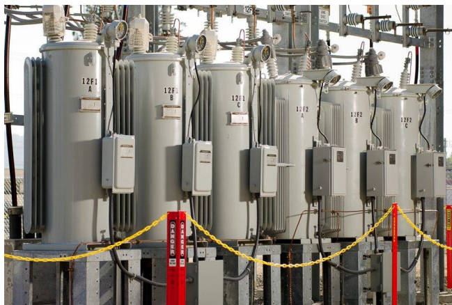
Substation voltage regulators
