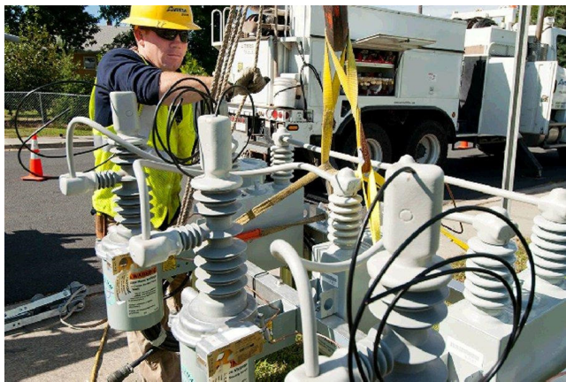
Capacitors banks for distribution lines
