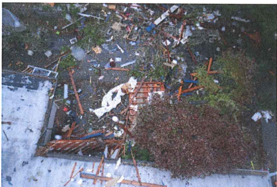
17. aerial view – debris blown into e.n. yard
