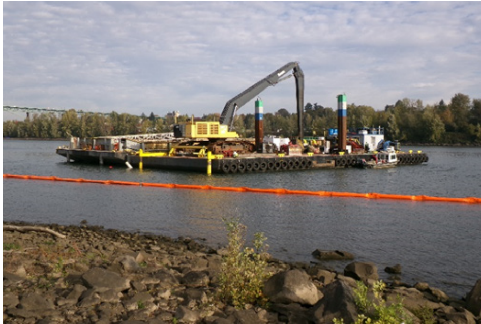
Excavator barge and swell materials removal barge staged at the site outside of construction area pending waste characterization results and eventual transport off site for disposal (10/31/2023).
