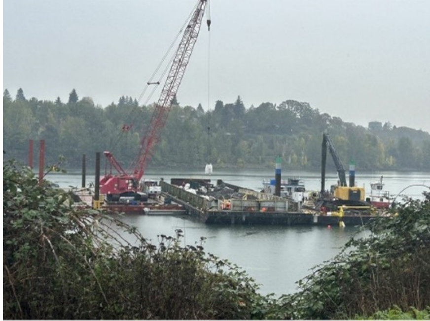
Flying 2-ton super sacks of Portland cement into swell materials removal barge (11/1/2023).
