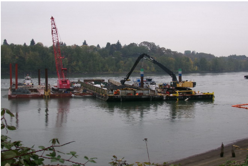
Mixing Portland cement in removed ISS-treated materials stored on Barge No. 7 and collection of 5-point composite sample for TCLP VOC analyses (11/1/2023).
