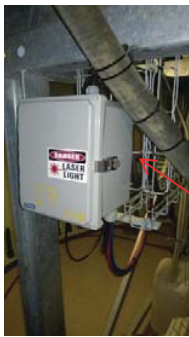
Turbine Fiber Distribution Panel - Located in basement of WTG
