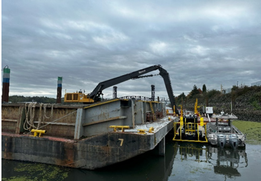
Performing leveling of ISS-treated surface to create an approximately level plateau for installation of the long-term sampling ports (10/23/2023).
