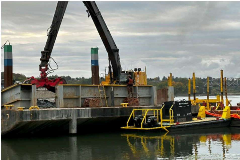
Mixing removed ISS-treated materials stored on Barge No. 7 and collection of 5-part composite IDW characterization sample (10/23/2023).
