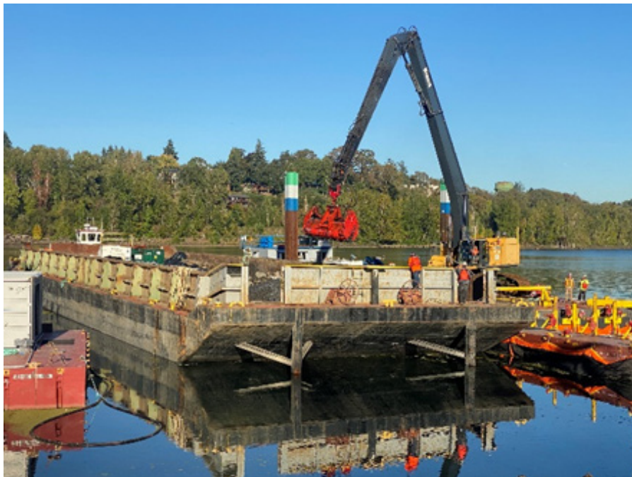
Performing ISS-treated surface leveling removal near rows 2 and 3. Swell material barge in foreground (10/18/2023).
