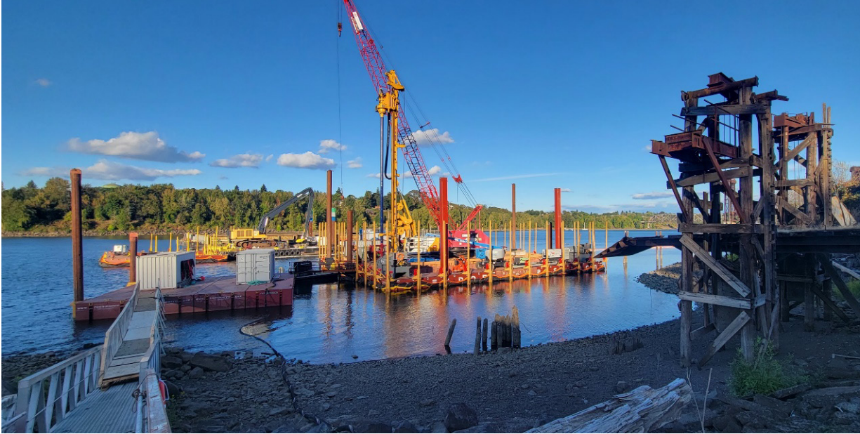
Project layout with ISS and swell material barges and associated equipment and gangway installed (9/20/2023).
