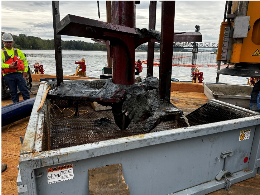
ISS drill rig auger bit after completion of column location 1-1. Excess material washed into shown watertight containment bin (9/23/2023).
