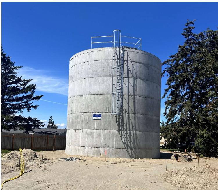
New Estates reservoir
