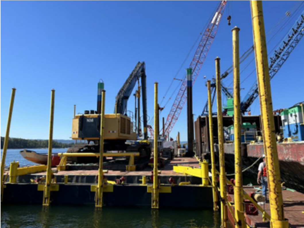
Installation of moonpool spuds and PC300 LF excavator on swell material removal barge (9/14/2023).
