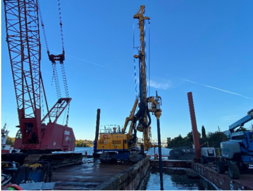
Performing ISS auguring at column 8-10. Refusal was encountered at 24.5 feet below ground surface (10/12/2023).
