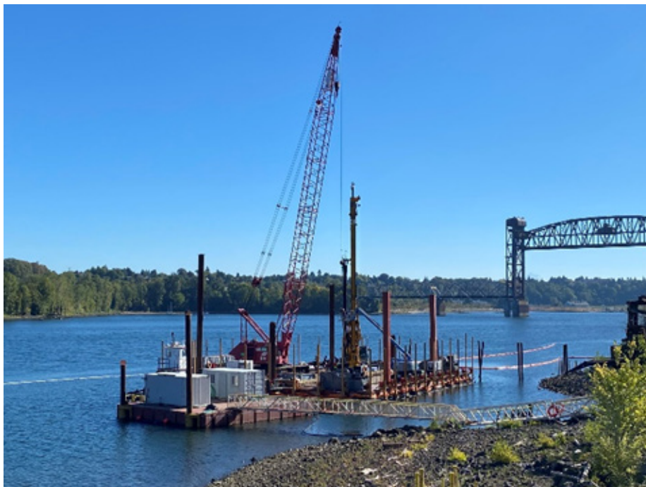
ISS drill barge and crane staged within Field Pilot Study area with environmental controls in place (10/05/2023).
