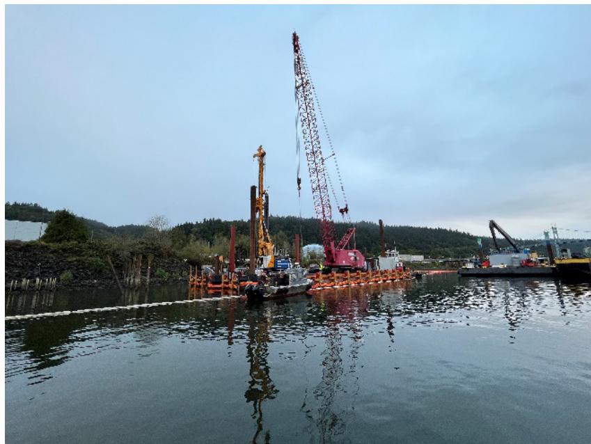
View of containment booms along south perimeter of the Field Pilot Study area (10/03/2023).
