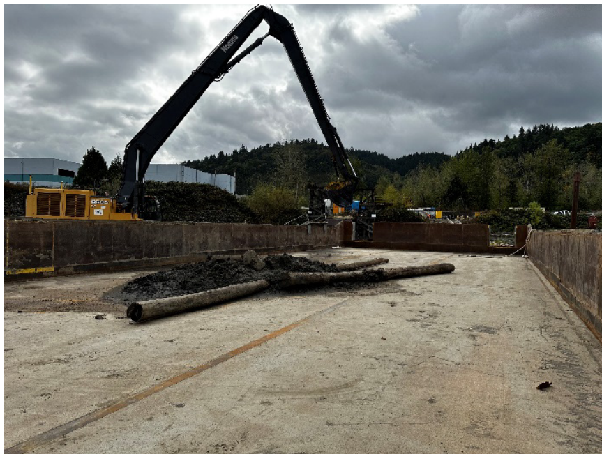
Swell material removal barge No. 7 prior to swell material removal at columns 1-4 and 1-9 (10/04/2023).
