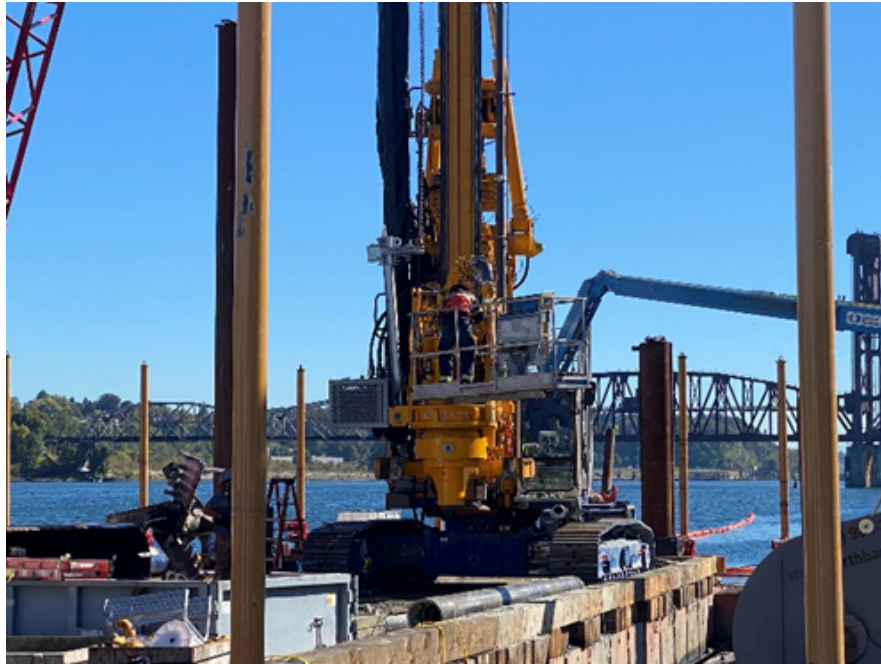
Reconfigured the drill pipe on ISS drill rig to facilitate drilling at deeper water depths (10/05/2023).
