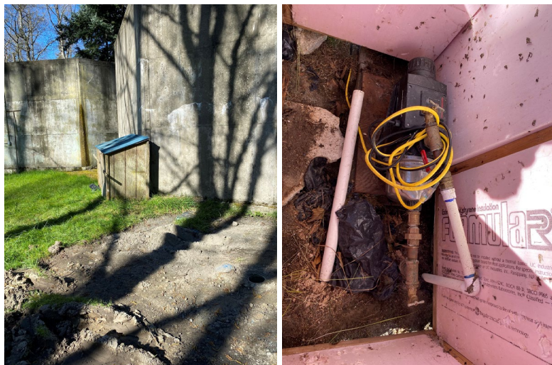
(L) Booster pump housing near reservoir (R) 1-HP Booster pump for 2 connections
