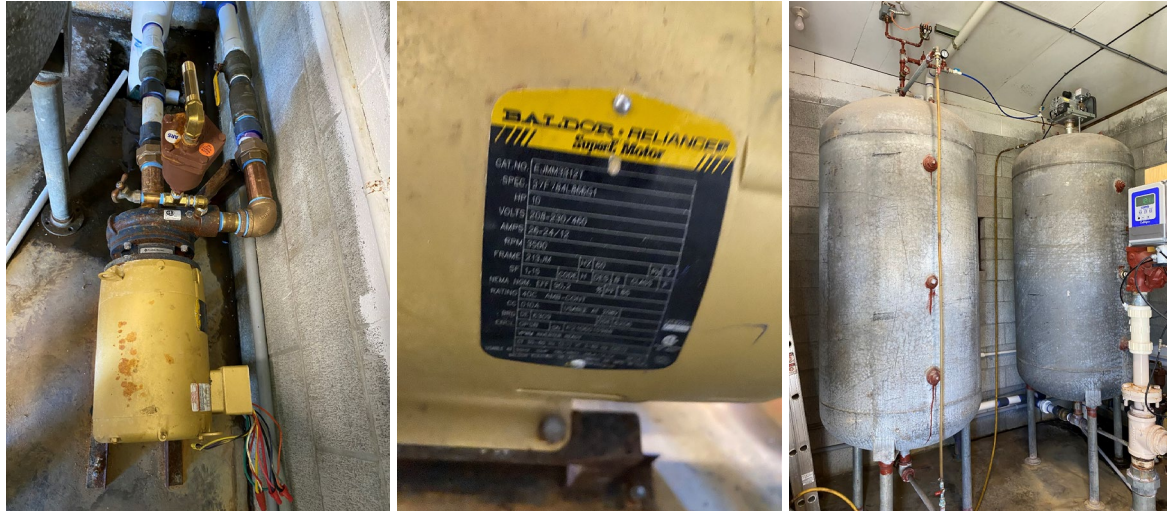
(L) & (Center) Booster pump at Fort Nugent site (R) 300-gallon pressure tanks at Fort Nugent site
