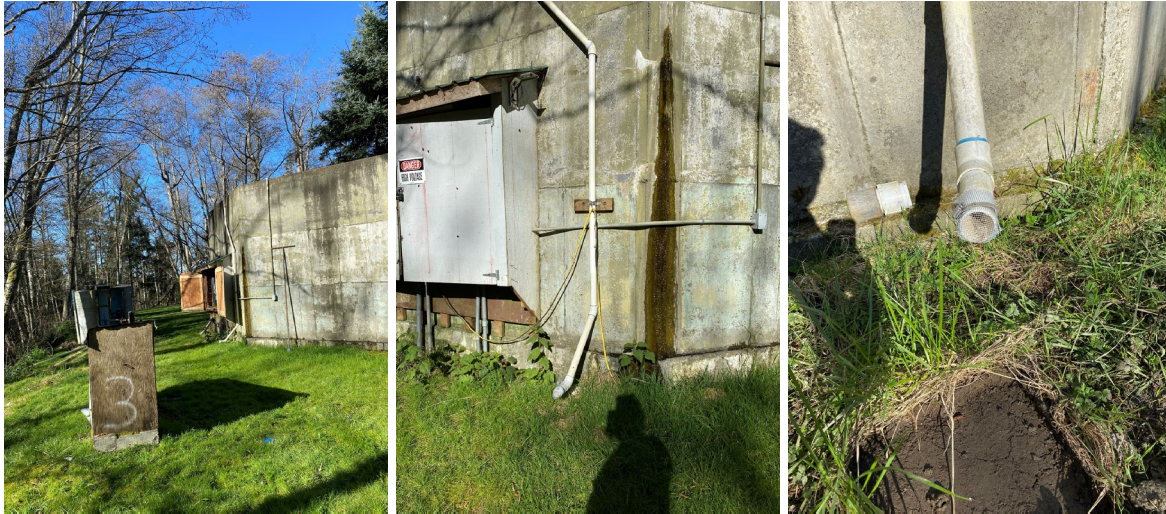
(L) Existing reservoirs with wells nearby (Center) Overflow for reservoir (R) Finer mesh needed for overflow screen
