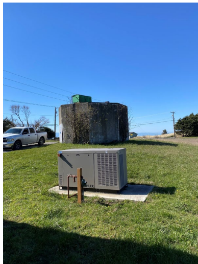
(Above) Generator at Fort Nugent site
