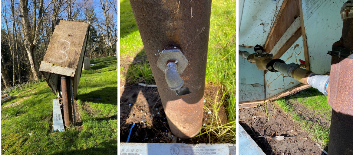
(L) Well #3 (Center) Secondary vent on Well #3 (R) Source meter and sample tap
