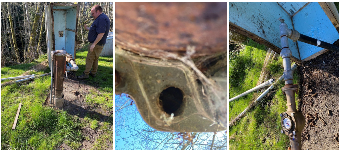
(L) Well #2 (Center) Screened vent on Well #2 (R) Source meter and sample tap
