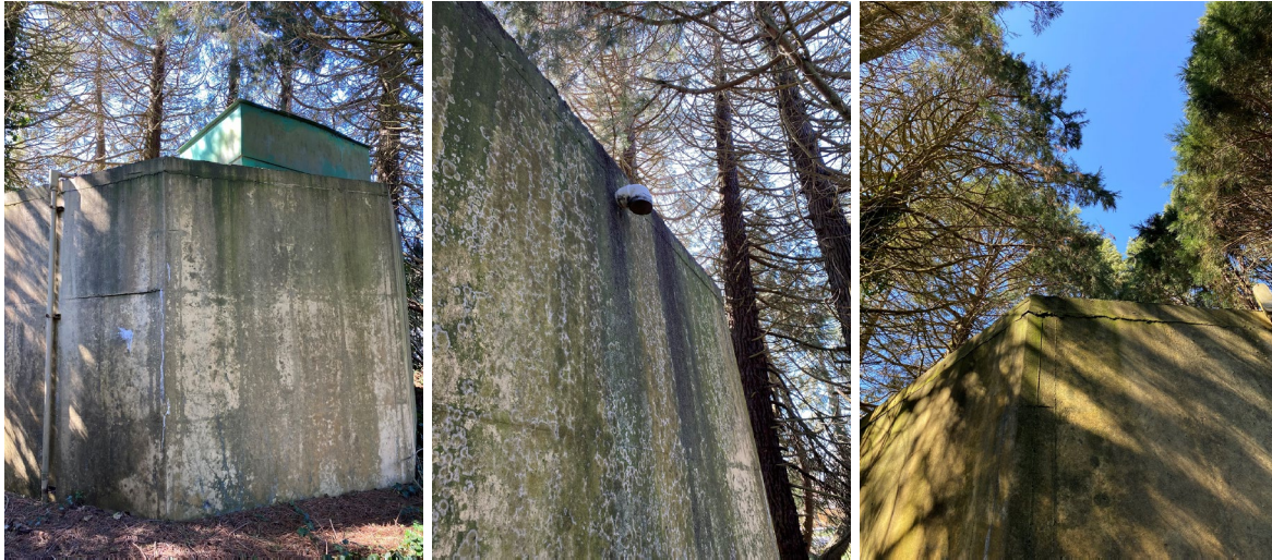
(L) Island View Reservoir (Center) Screened overflow at Island View reservoir (R) Trees overhanging the reservoir which results in excess debris on top of the reservoir
