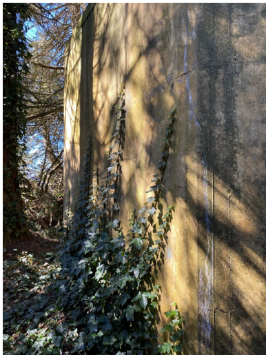
(Above) Vines growing up reservoir – can impact the integrity of the reservoir
