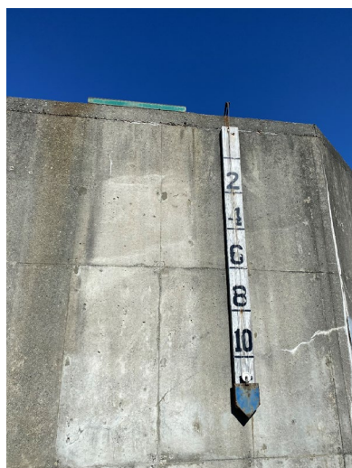
(Above) Fort Nugent tank-level device
