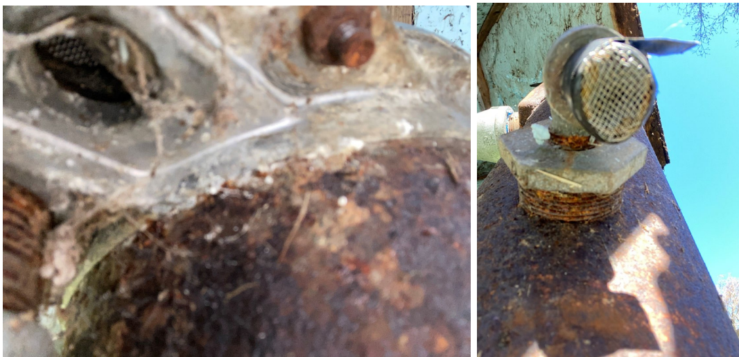
(L) & (R) Screened vents on Well #3
