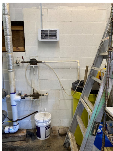
(Above) Chlorine and potassium permanganate solution tanks and chlorine injection point
