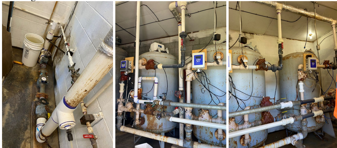
(L) Chlorine injection point (Center) & (R) 3 Greensand media filters
