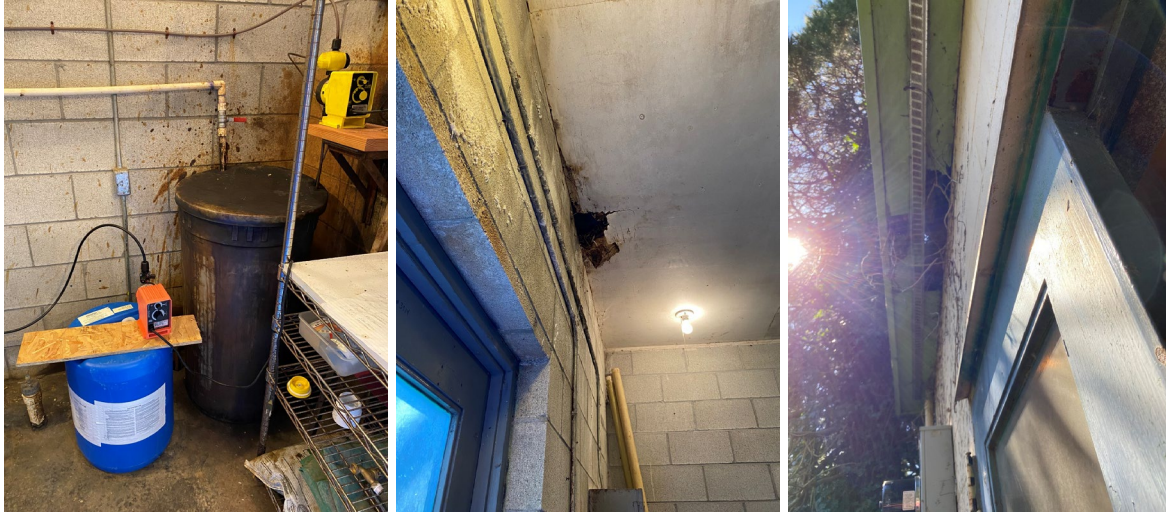
(L) Potassium permanganate and chlorine solution tanks with feed pumps (Center) & (R) Rot in the ceiling of treatment house – needs major repair.
