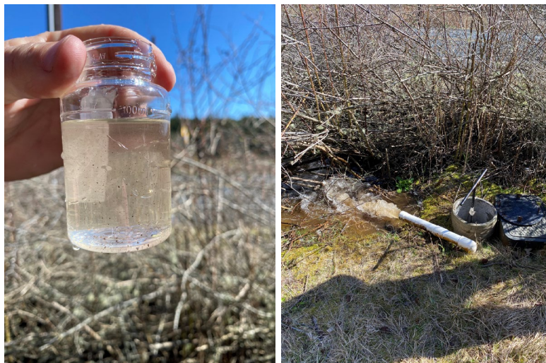
(L) Visible manganese particles in flushed water (R) Flushing of main near Fort Nugent site
