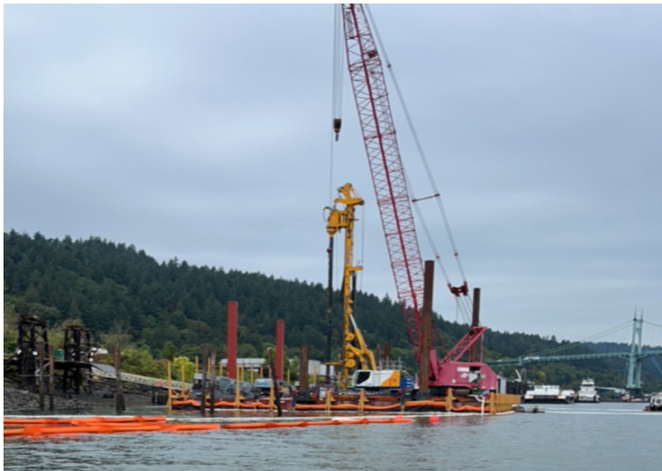
View of ISS drill rig barge from water quality monitoring station EW-1S (09/27/2023).
