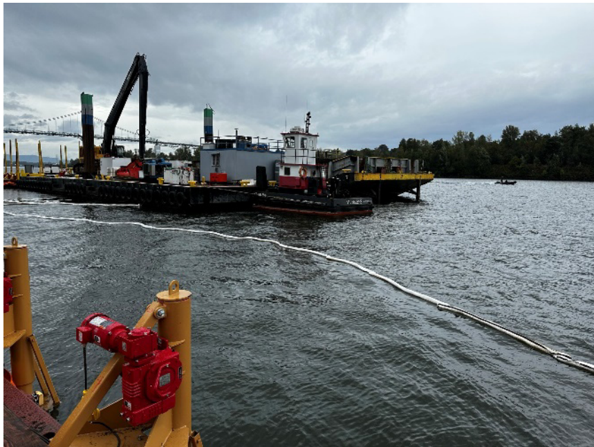
Channelward oil absorbent boom installed and connected to the anchored downriver and upriver oil containment booms and swell removal barge. This additional boom results provides oil containment surrounding the entire perimeter of the larger work area and will be maintained for the remainder of the field pilot study (09/25/2023).
