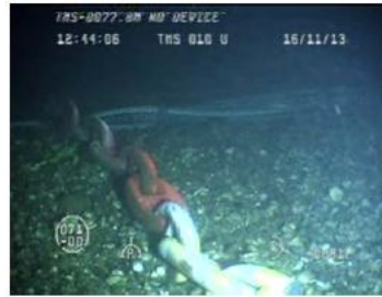
Figure 9 - Anchor Chain on Splice Box
