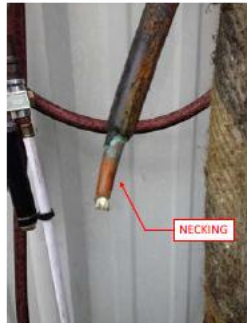
Figure 23 - Necking on Copper Sheath
