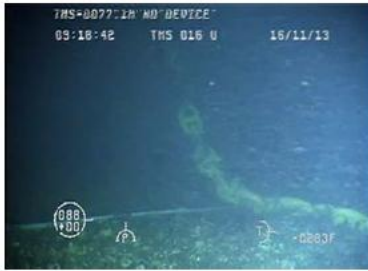
Figure 10 - Anchor Chain on Cable
