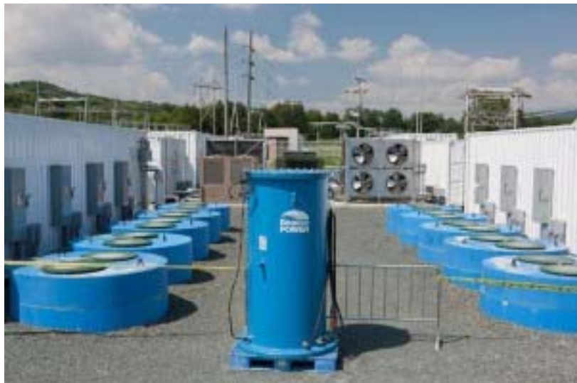
Figure 23- Smart Energy 25 100 kW / 25 kWh
