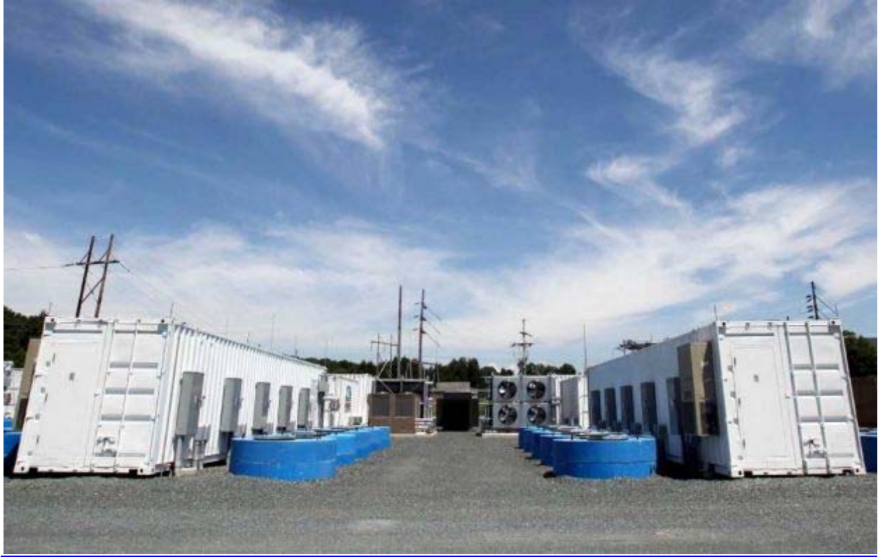
Figure 24- Flywheel Plant New York
