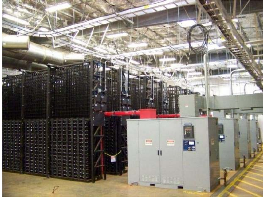
Figure 15- PowerCell™ Stacks with PCS
