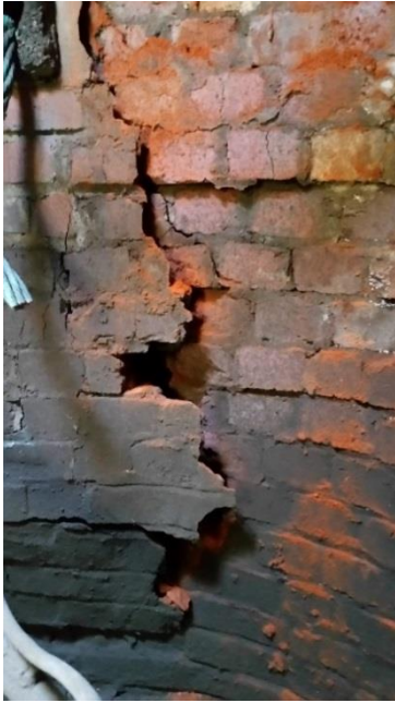
Figure 25, Interior of a badly deteriorated old manhole in a heavily traveled street
