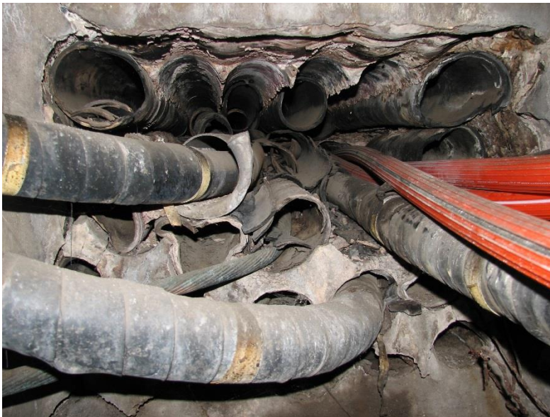
Figure 26, Duct bank damage entering an old deteriorated manhole
