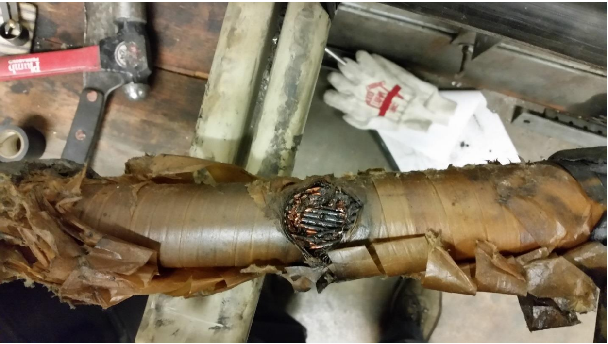
Figure 23, A second faulted PILC cable
